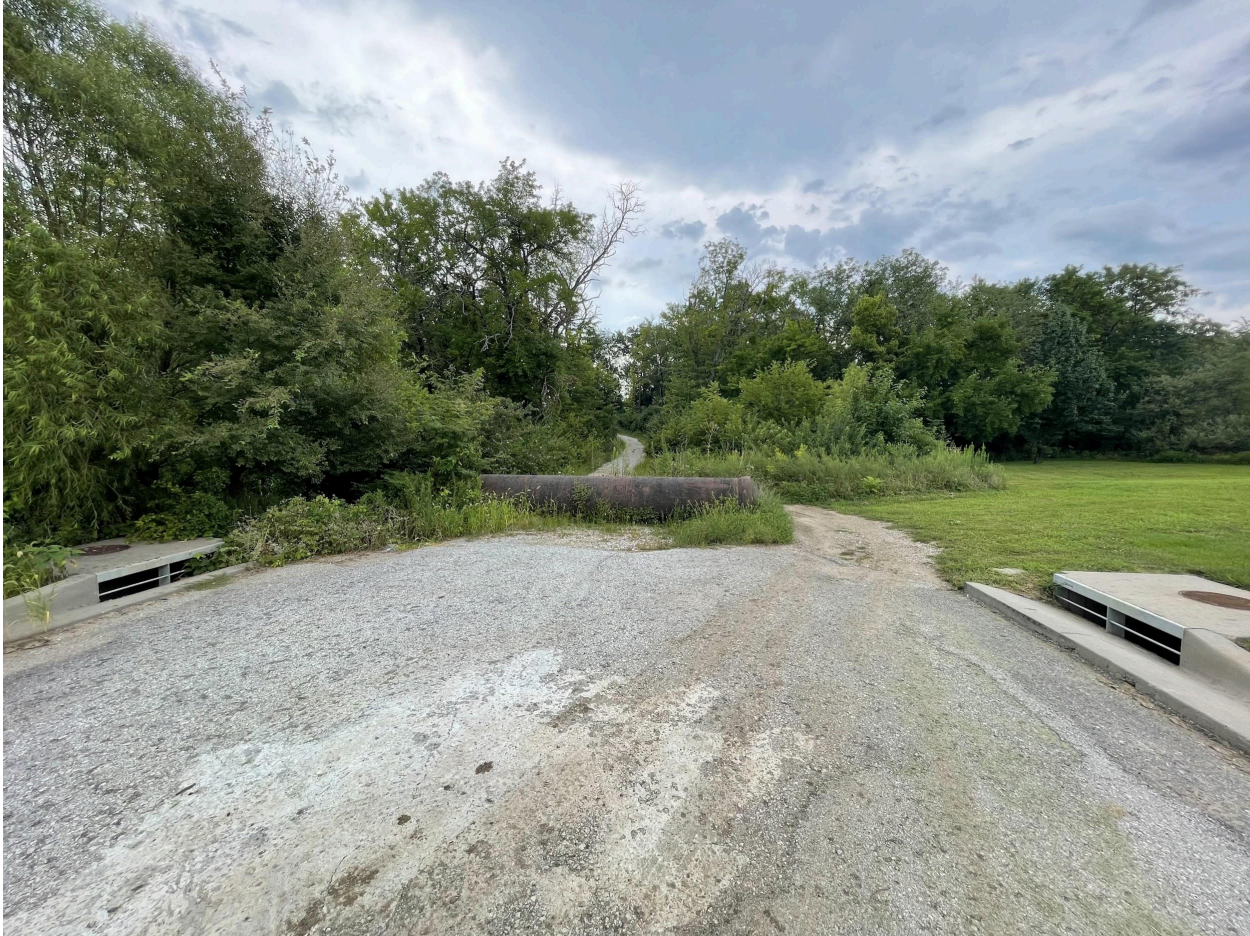
Looking SE at the Terminus of Creekmoor Drive South of Rannoch Ln
